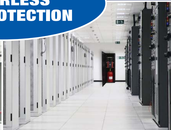
Large Room Protection
